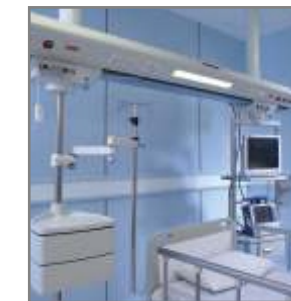
Ceiling Supply Beams
